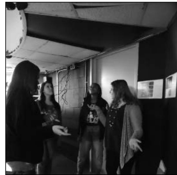
Students from Mr. Hudkins' drama class check out the fix Mr. Bamburger did to the ceiling where tiles fell out.
