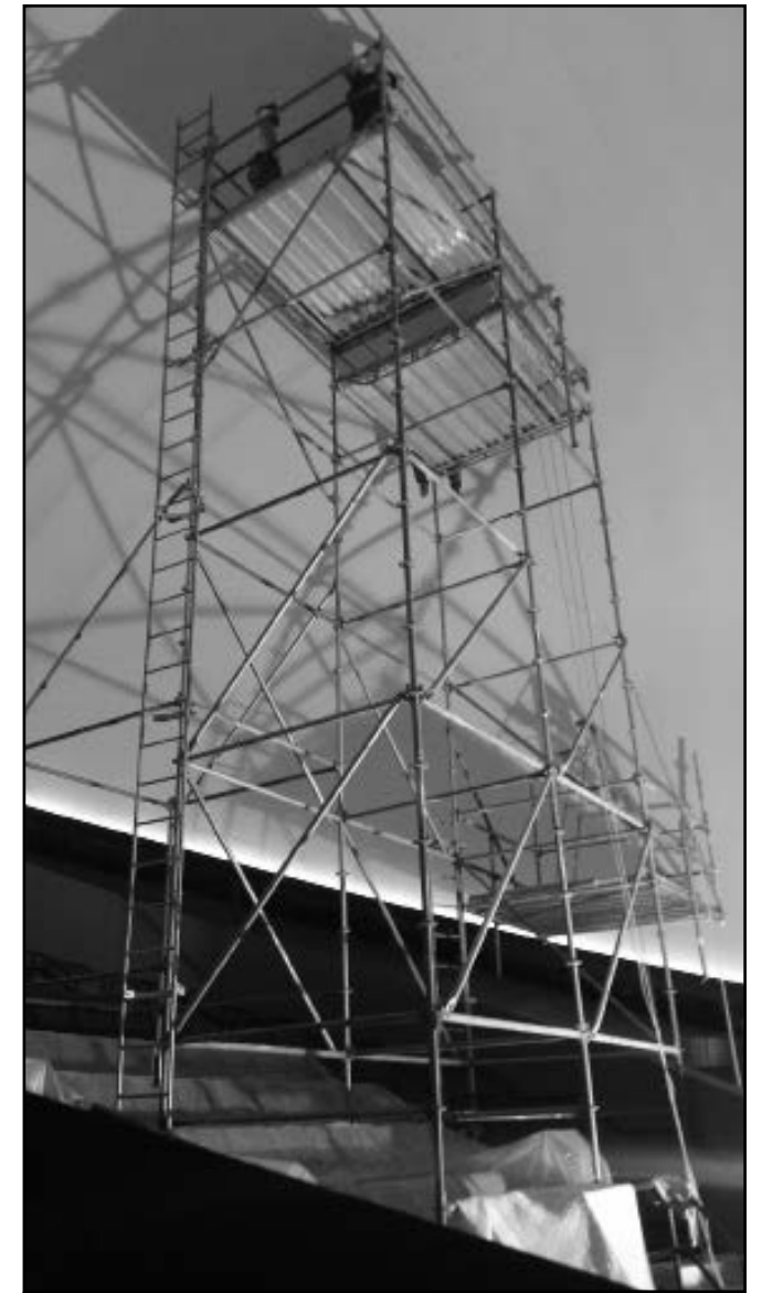
Getting to the panels at the top of a tilted 55-foot dome is no small feat!
